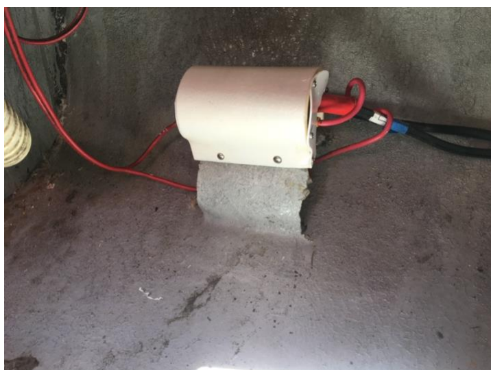
Almost completed installation. Not shown are the 3 wire clamps I made from the portion of the pipe I cut out. I heated and formed the 4" strips into clamps to hold the wire. They were 5200'ed onto the hull.
