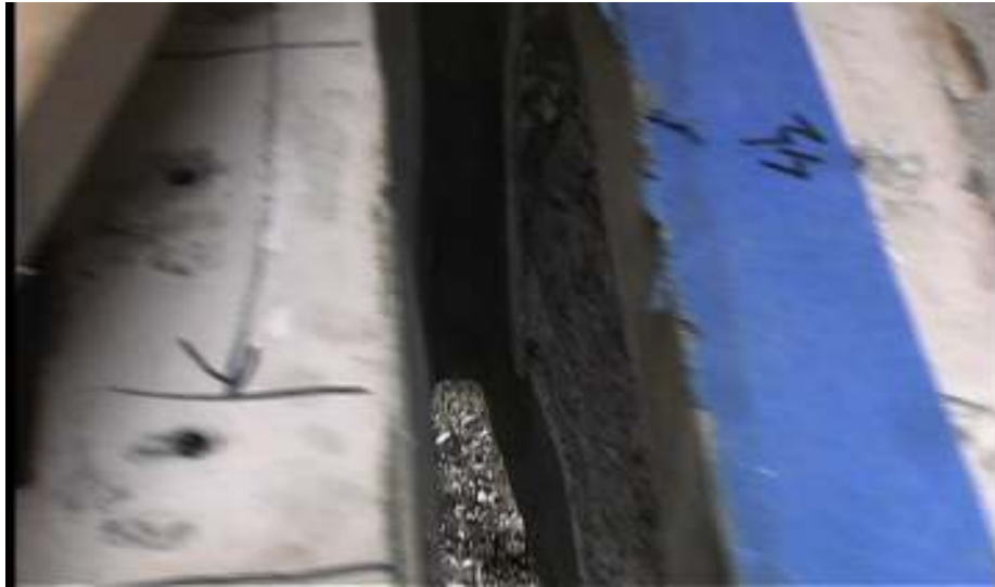
The aft port side hole in my trunk.. seeing the cement was always a frightening site when coming back to work on the project.
