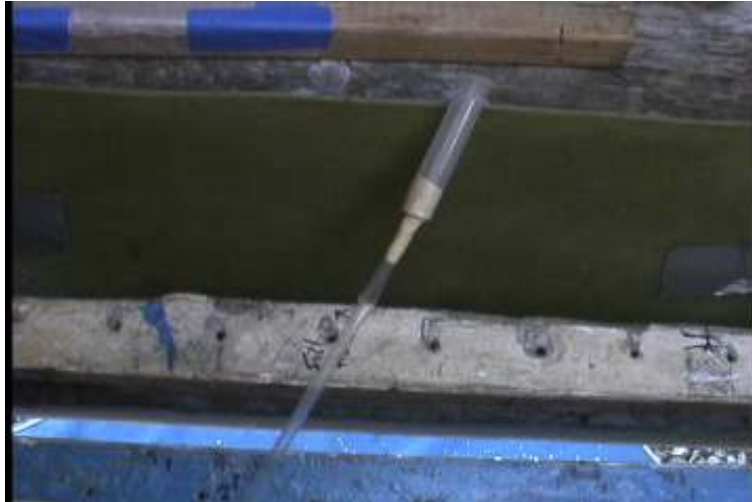
One of the more difficult tasks: injecting the thickened epoxy into voids between the new panels and the trunk wall.
